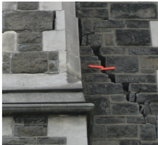
Figure 1: South transept wall, January 14, 2013
